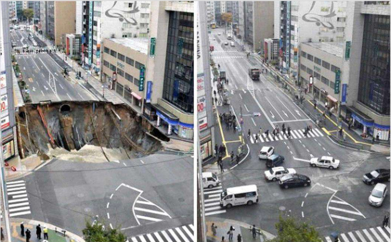
Photo of a giant sinkhole (L) measuring around 30 metres (98 feet) wide and 15 metres deep, which appeared in a five-lane street in the middle of the Japanese city of Fukuoka on November 8, 2016 and of the same section of road (R) after repairs were made on Nov.15
