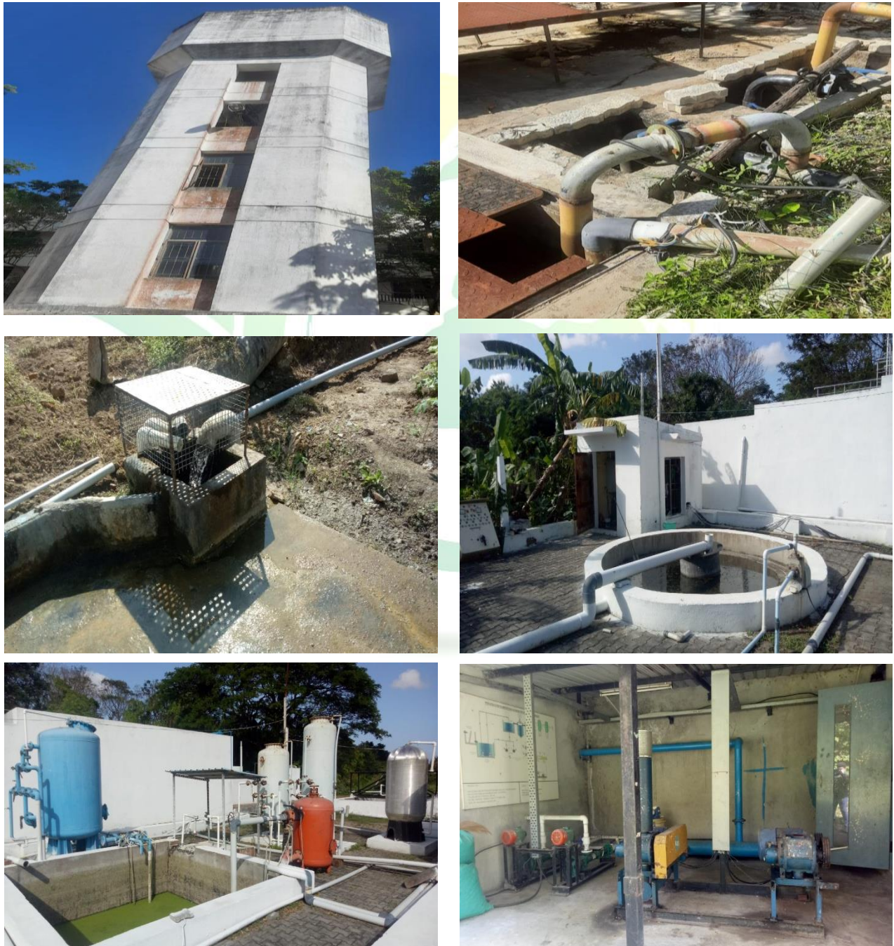
Figure 14: Pumping system in the campus
