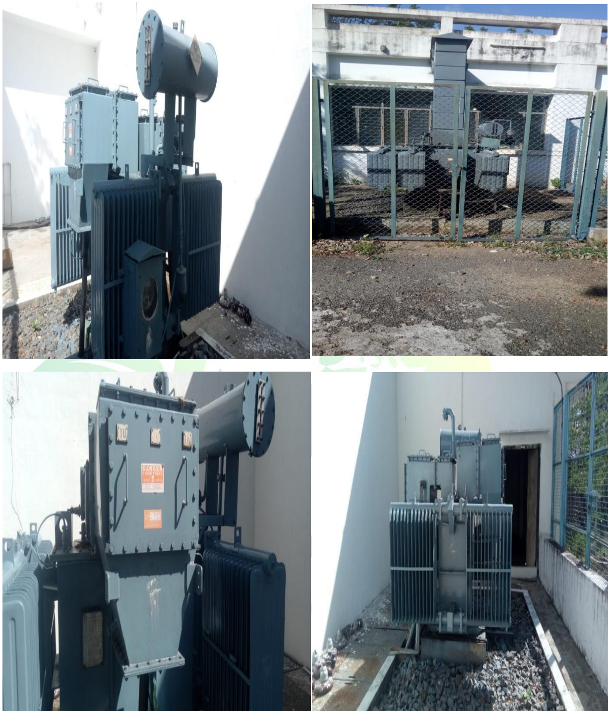
Figure 17: Transformer in the campus
