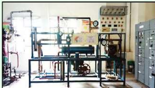
Steam Boiler Turbine Unit
