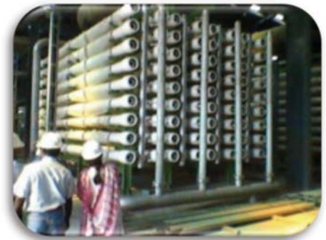
Dr.V.Rajini, Prof/EEE visiting the Desalination Plant at VadaNemili under construction by WBAG- Israel along with L&T team
