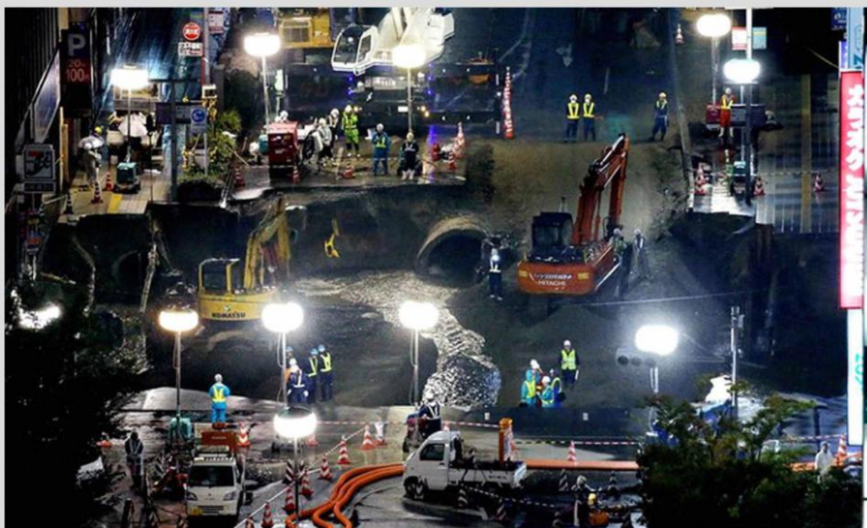
Work went on through the night to repair the huge sinkhole that formed in front of JR Hakata
